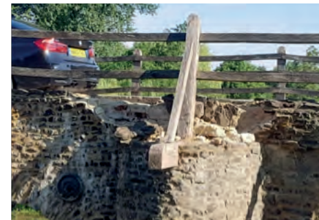
Rotted damaged timber
